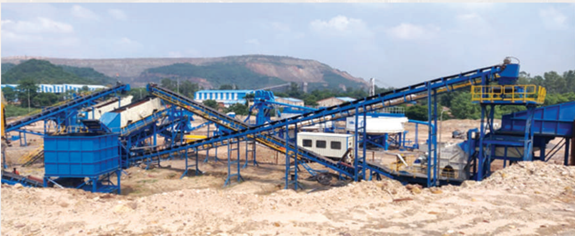
Amlohri Plant, NCL
