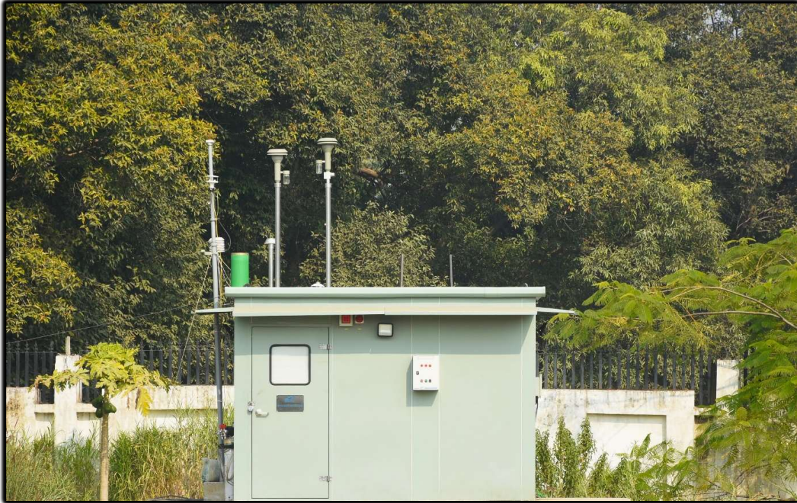
Picture: 01 CAAQMS Installed
