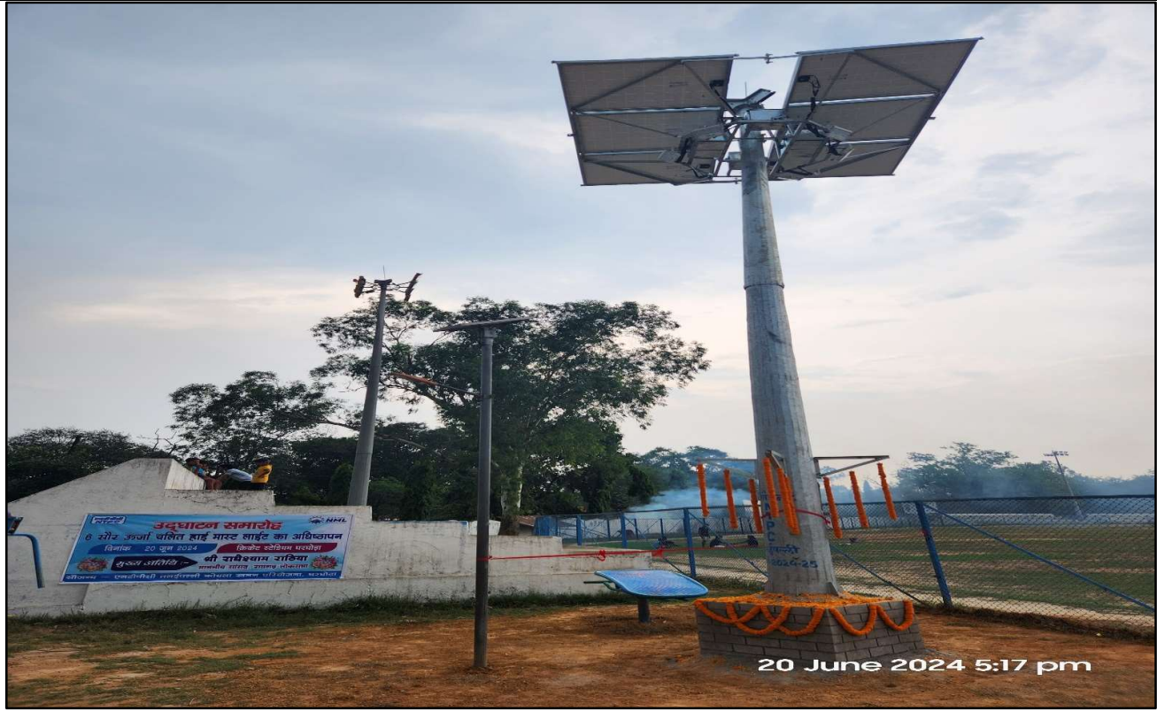
Inauguration of High mast Light at Gharghoda Stadium.
